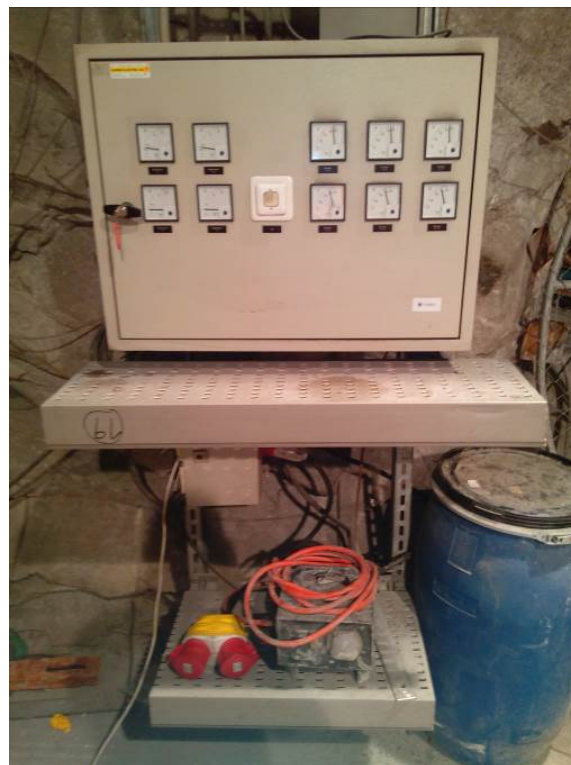
Fig. 6: Double headed three-phase connector below power cabinet.
