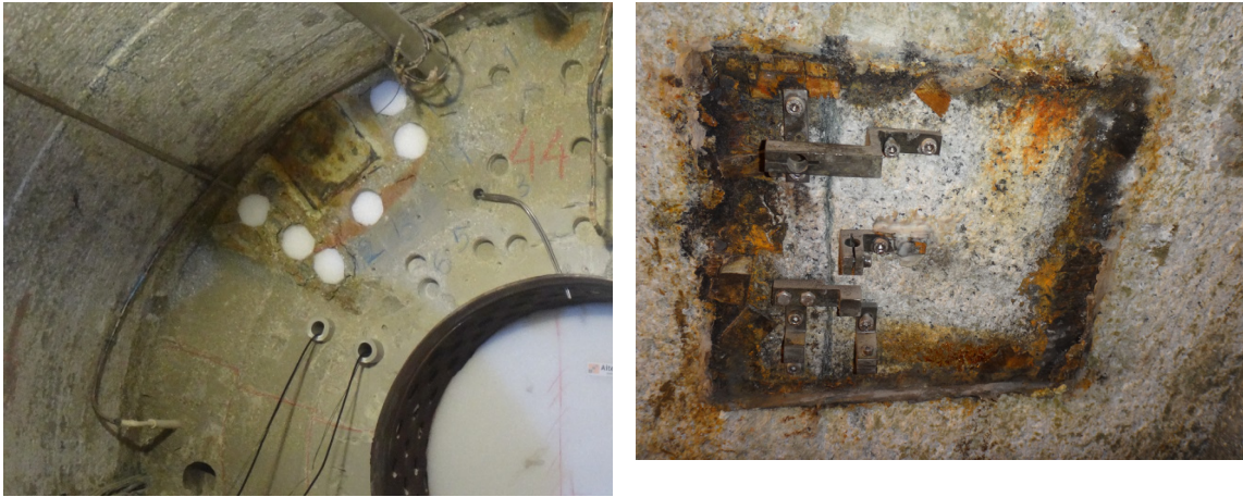
Fig. 65: Left, samples taken around fisurometer. Right, view of fisurometer location once the protective cap has been removed.
