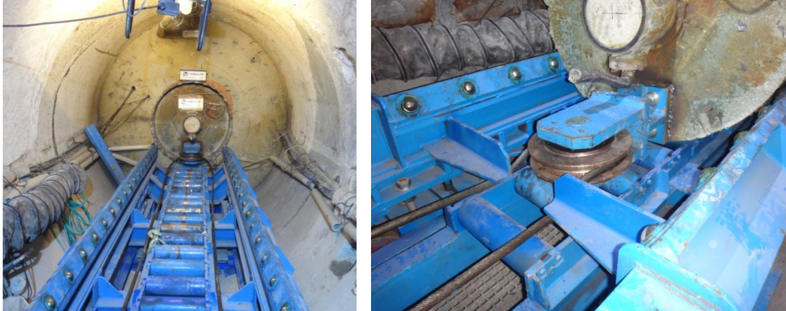
Fig. 48: View of the extraction car already positioned for the extraction manoeuvre (at the left) and detail of the return pulley installed at the heater front (at the right).
