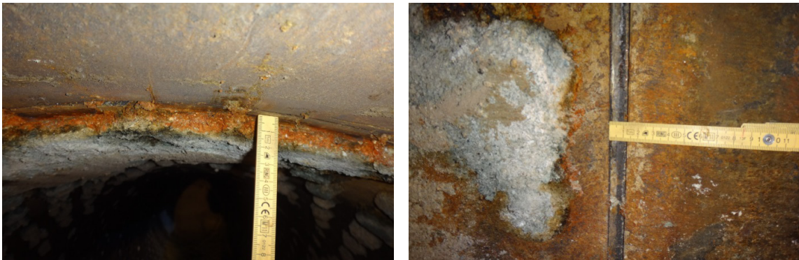
Fig. 52: Measurements made on the liner segments were the heater was placed and on the previous one.
