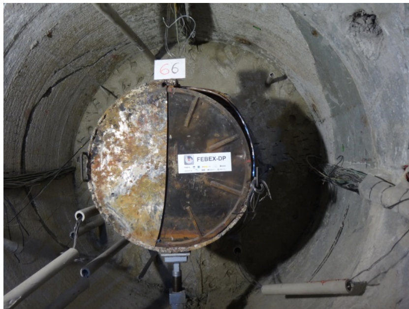
Fig. 34: Steel support for the dummy canister.
