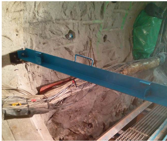
Fig. 7: Laser frame installed on lateral fixing on the gallery's walls.
