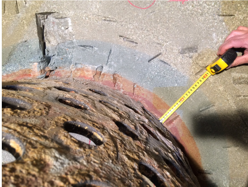
Fig. 44: Details of the colour aureoles of Fe-oxidation/reduction fronts close to the liner.
