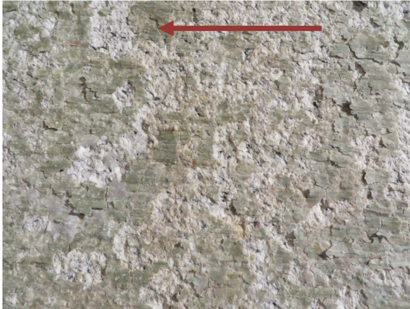
Fig. 40: View of longitudinal marks on the bentonite layer adhered to the gallery.
