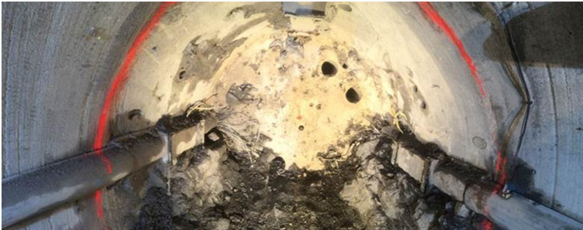
Fig. 22: Detail of the excavation advance and the impermeable mat at the rear of this first part.
