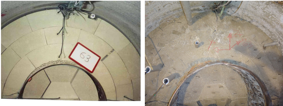
Fig. 41: View of bentonite layer 63 after installation (left) and during removal (right), Section 41.
