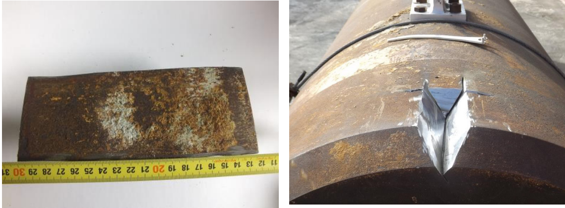
Fig. 63: Metallic sample from heater in Spain.
