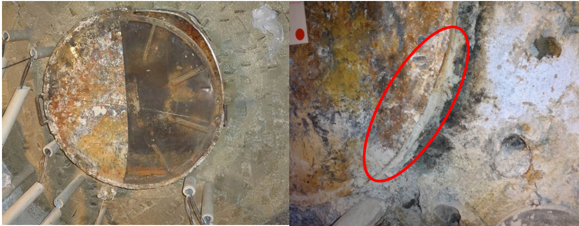
Fig. 33 View of the "dummy canister" (left) and its adhesion to the liner segment (right).
