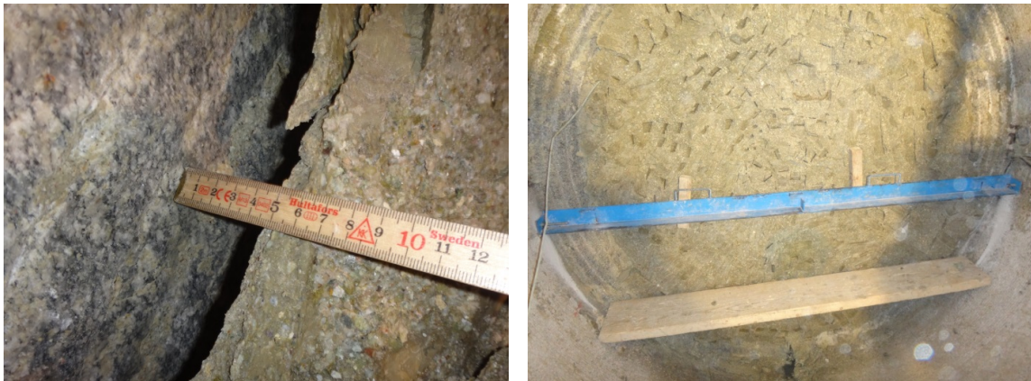
Fig. 58: View of the bentonite detachment at the end of the gallery.
