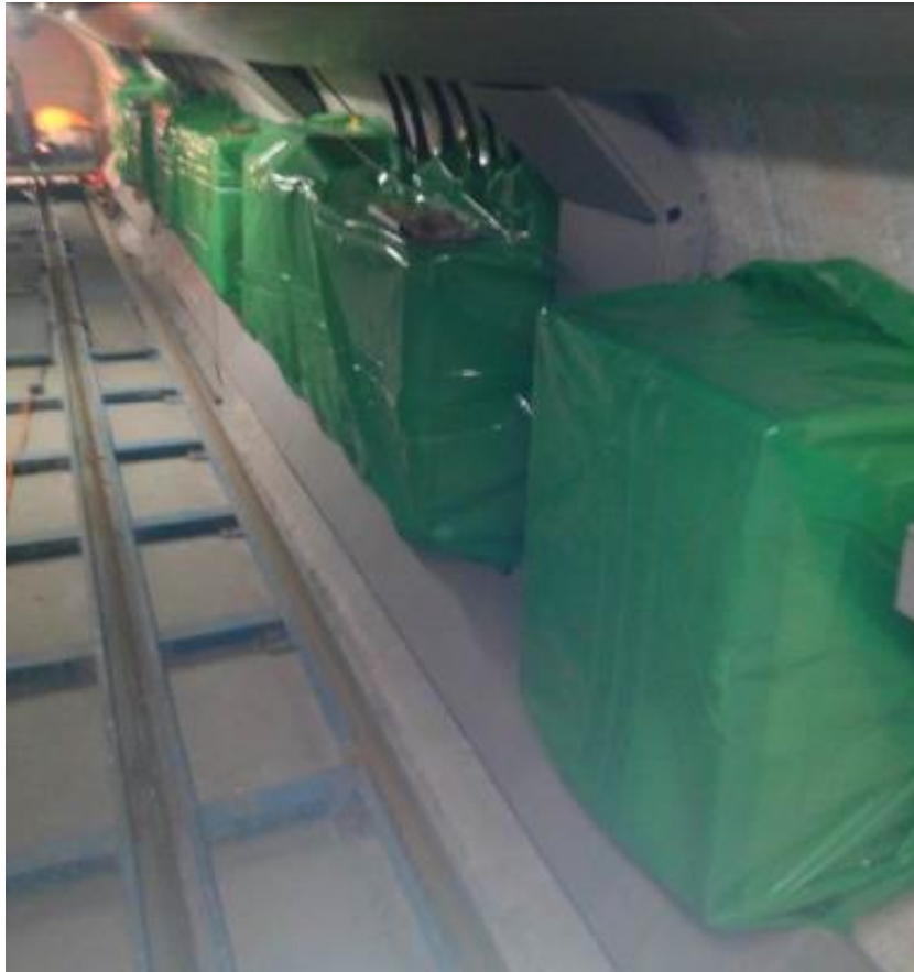
Fig. 12: Cabinets protected with a plastic sheet.
