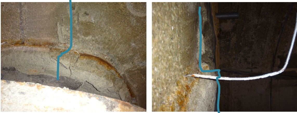
Fig. 56: Views of the insertion of inner blocks inside the last liner segment. The blue line shows the step between outer blocks and inner blocks.
