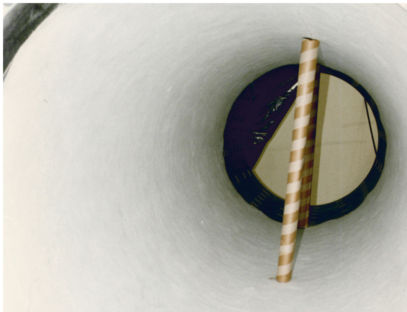
Fig. B-3: Installation of geotextile layers in the Mock-up Test structure prior to bentonite emplacement.
