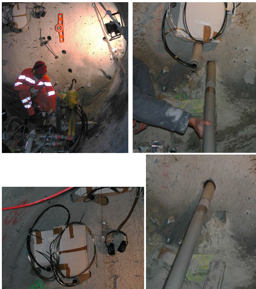
Fig. 29: Drilling of boreholes and insertion of the six C_x pipes for water sampling in May 2003
