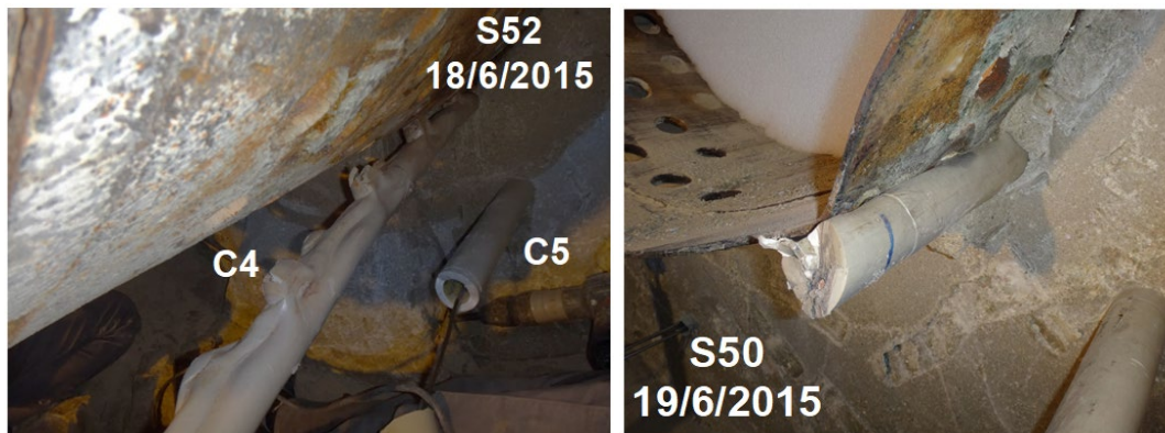
Fig. 56: Visual aspect of the pipe C4 from Section 55 to Section 45 (from the frontal part to centre of the heater): deformation probably due to thermal stress by overheating
