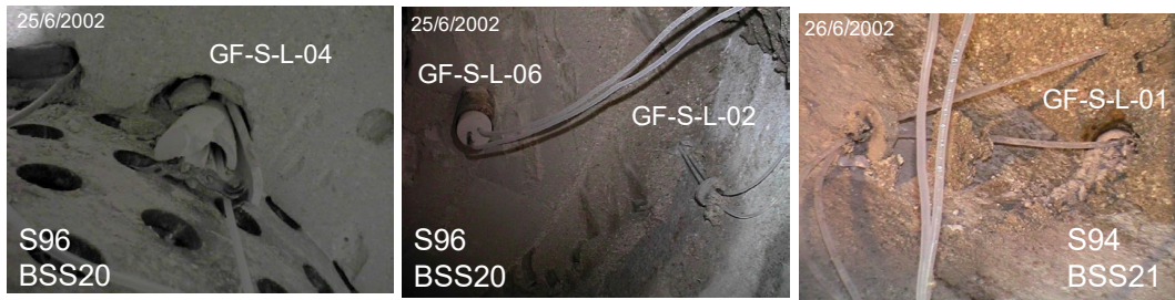
Fig. 48: Visual aspect of the GRS pipes during the dismantling of the Heater #1: bentonite Slice 96 (BSS20, Instrumented Section L) in 25 June 2002, and Slice 94 (Bentonite Sampling Section BSS21) in 26 June 2002
