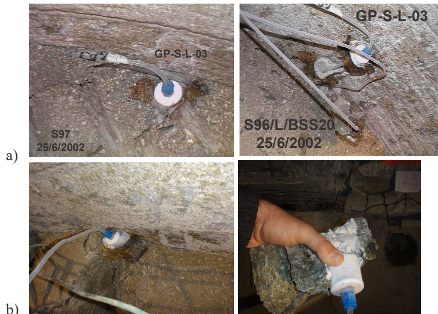
Fig. 49: Visual aspect of the GRS pipes for water pressure measurements during the dismantling of the Heater #1: a) GP-S-L-3 in the bentonite Sections 96 and 79 (Instrumented Sections L and M1, respectively). b) GP-S-H-3 for pore pressure measurements during the dismantling of the Heater #2 (29/5/2015) in the Slice 63 (BSS40, Instrumented Section H)
