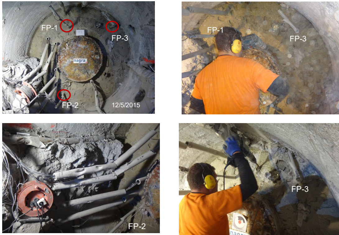
Fig. E-8: First visual position of the PP-H 100 tubings of the gas pipes taking inside the four 1/8" SS sampling tubings at the bentonite Slice 74 (Sampling Section 36, Instrumented Section P) in contact with the concrete plug (12 May 2015)
