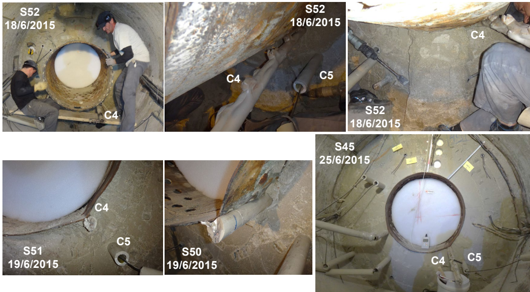
Fig. E-24: Visual aspect of the pipe C4 from Section 55 to Section 45 (from the frontal part to centre of the heater): deformation probably due to thermal stress by overheating
