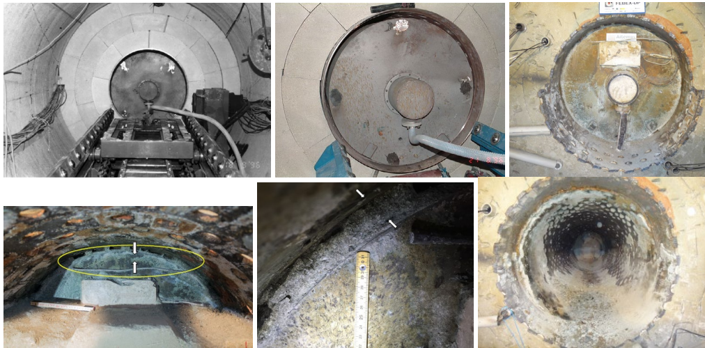
Fig. E-17: Visual aspect of the heater prior and after the FEBEX in situ test
