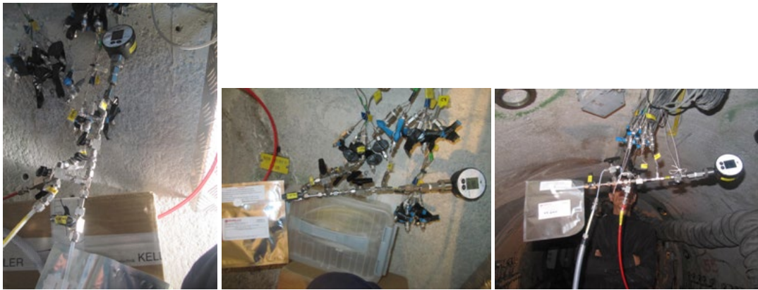
Fig. 102: Collection of porewater in the August 2014 sampling campaign from the pipes located: a) at the right side of the gallery, b) at the left side of the gallery and c) at the top of the gallery
