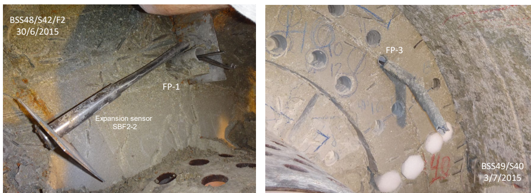
Fig. 53: Visual aspect of the stainless steel pipes with no evidences of external corrosion
