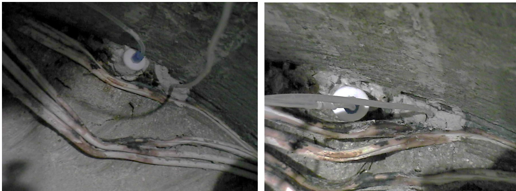
Fig. E-2: Visual aspect of the GF-SL-03 pipe during the dismantling of the Heater #1 from the Slice 79 (S79) or Bentonite Sampling Section 29 (BSS29) in 10 July 2002
