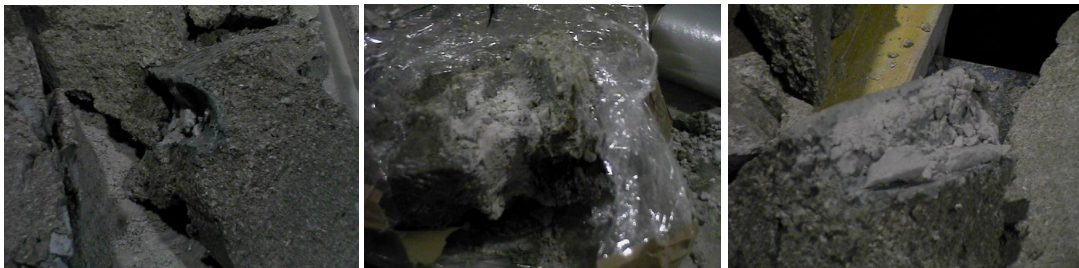
Fig. E-3: Visual aspect of bentonite blocks from Section 20 (Slice 96, Instrumented Section L), showing a bentonite greenish halo around a broken ceramic pipe
