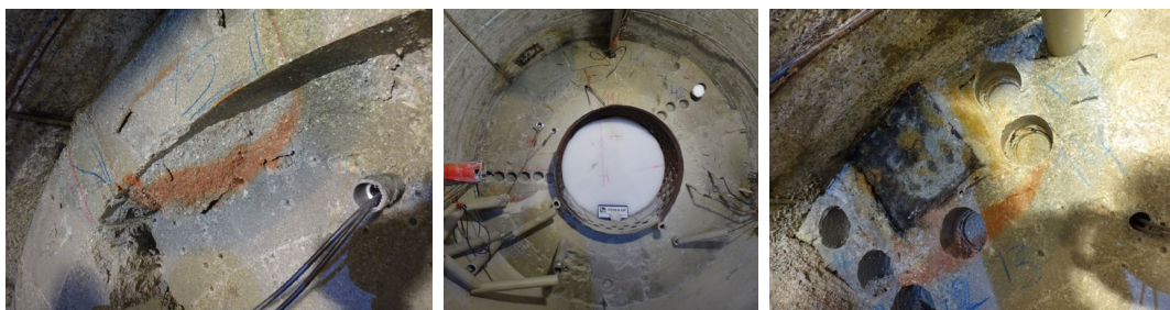
Fig. 83: Influence of the corroded fissurometer from bentonite Section 47 to Section 40, which was located close to pipe FP1
