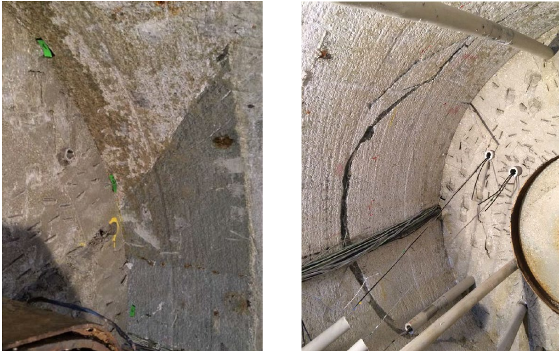
Fig. E-21: a) Gallery at ~ 3 o'clock showing interface of granite/lamprophyre and contact to bentonite further to the left (Section 37). b) Galleries' left side, detail lamprophyre under "Part B, Structure 5" (Section 39)
