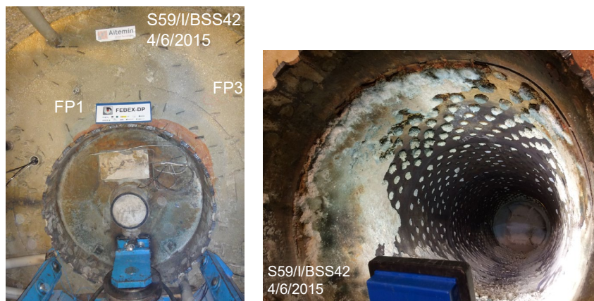
Fig. 50: Location of pipes FP-1 and FP-3 around the Heater # 2 (carbon steel) and visual aspect of the internal part of the liner during dismantling
